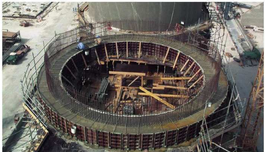
Silofundamente, BRN-Bahrain; Fa. Güllermark TR-Türkei & Mannai BRN-Bahrain
